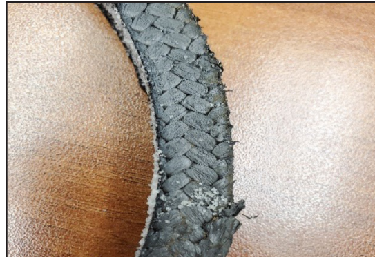
Damaged packing ring saturated with brine.
